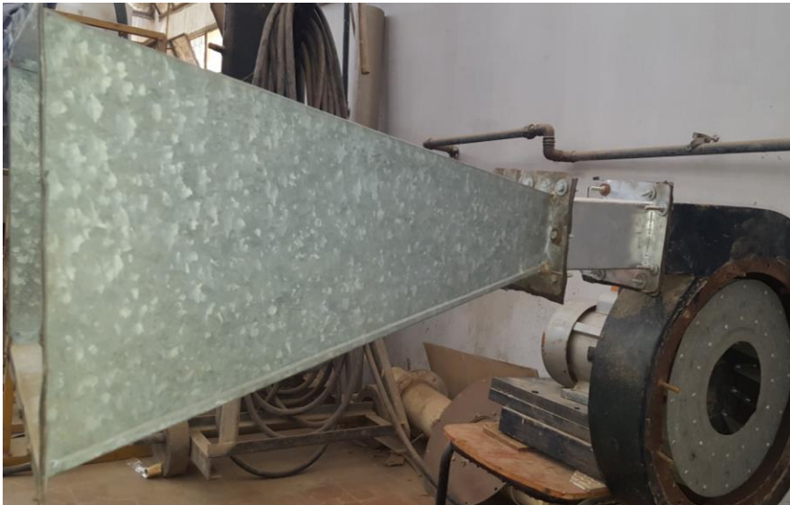
Fig. 4. 2 Air Supply Section
